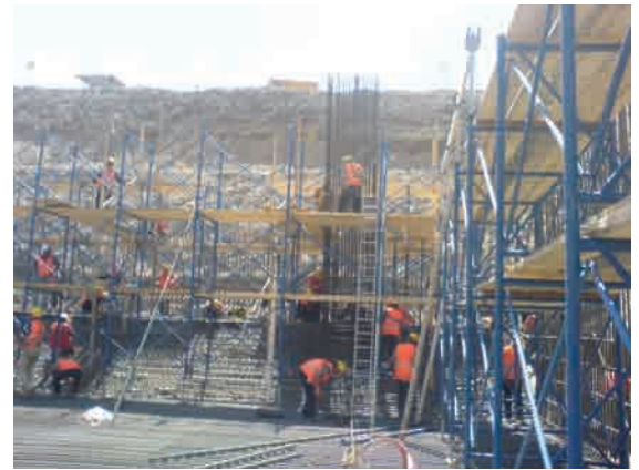
MKH Shoring Frames used as access scaff at the massive foundation job of a high-rise building at Almaty, by ENKA
