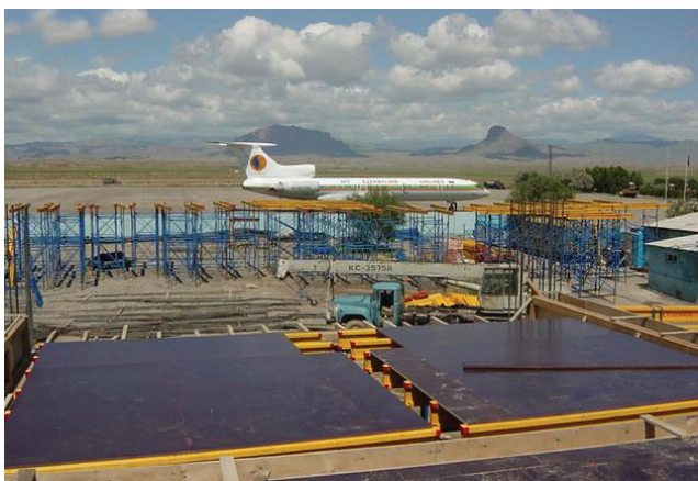
"Nakhichevan Airport" project has been completed with MKH 150 Tables in record time, by ERENPORT
